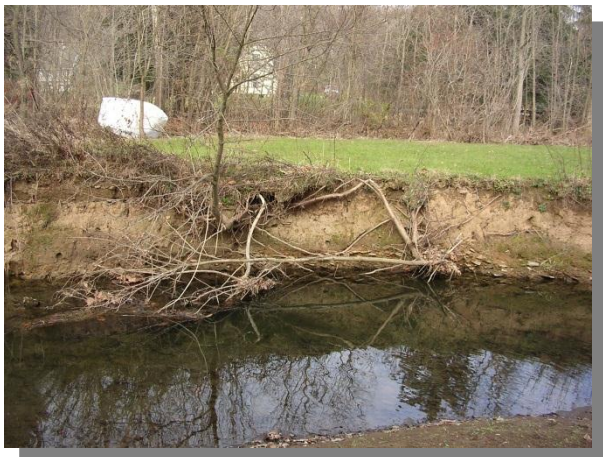
Environmental Detriment along Plum Creek
