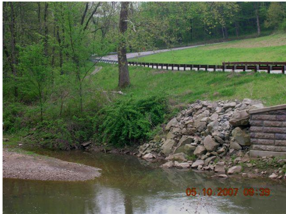
BEFORE – Haphazard repair of streambank erosion; sediment deposits in watercourse
